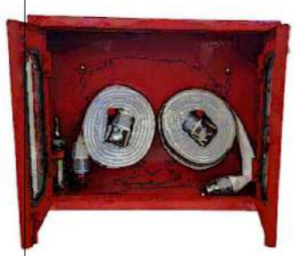
FIRE FIGHTING HYDRANT BOX
