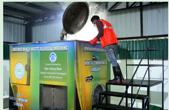
Decentralised Waste Processing Plant
