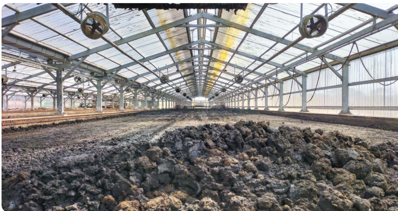
Picture-Solar sludge dryer at Goa for preparation of FOM
