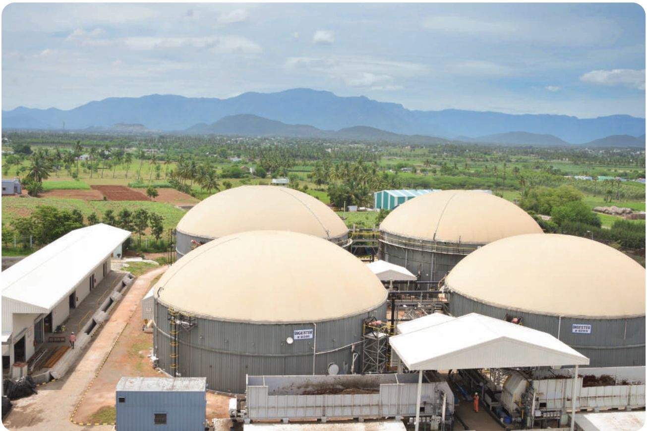
Picture—Fixed-dome Gas Holder at Namakkal CBG plant
