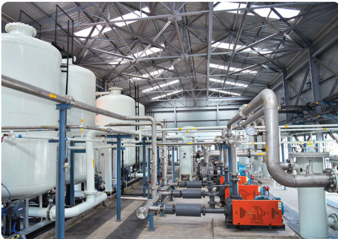
Picture-Purification System at Namakkal CBG plant
