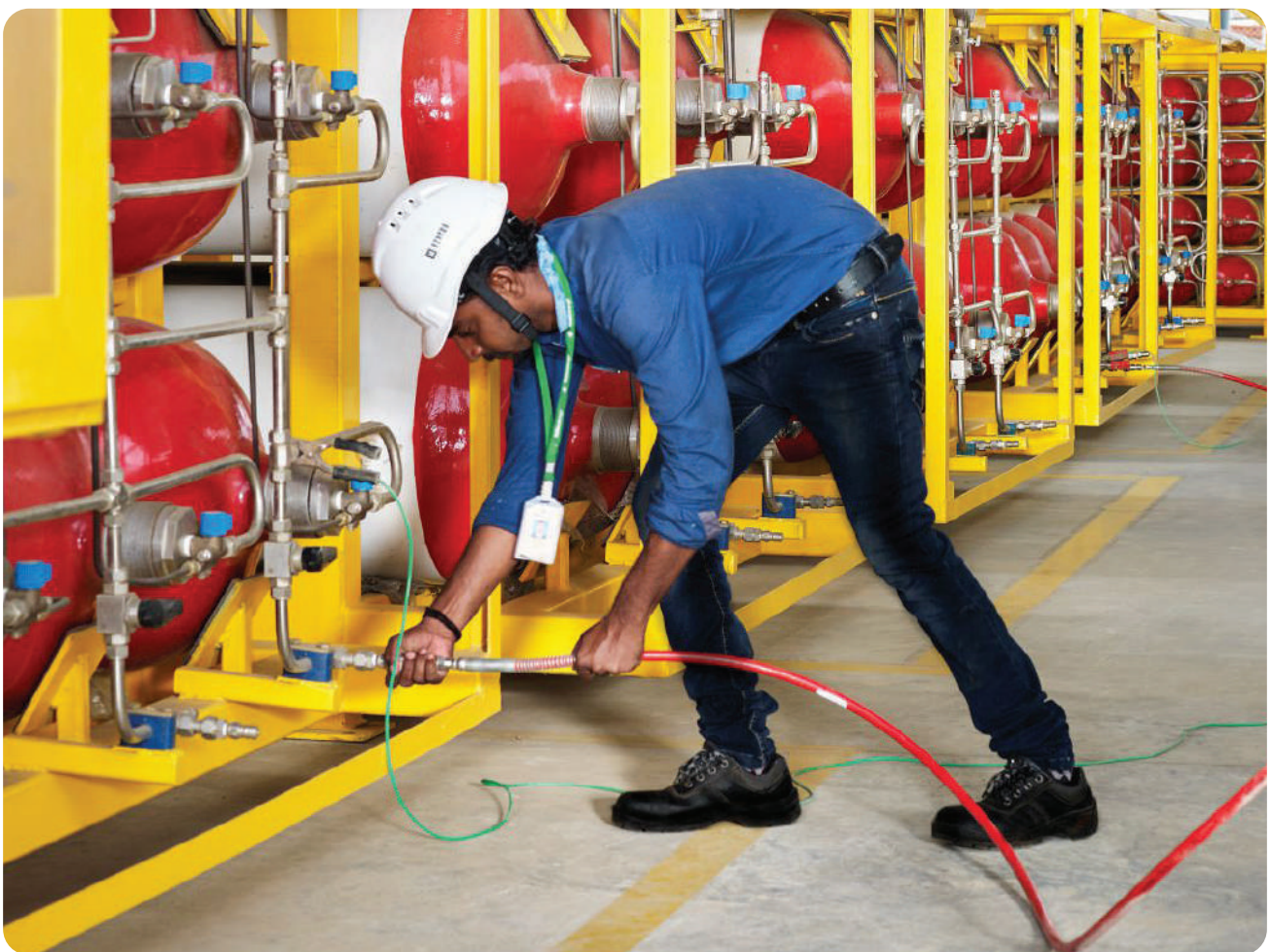
Picture-CBG Cascade at Pune CBG plant
