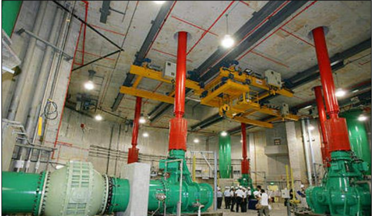
Influent pumping station at Changi Water Reclamation Plant. The 50 m deep has two pumping stations and a coarse screen shaft ( https://www.water-technology.net/projects/changi-reclamation/ )
