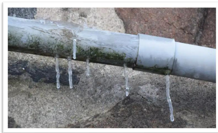
Fig. 1.4: Frozen Sewer Pipe in Colder Region
