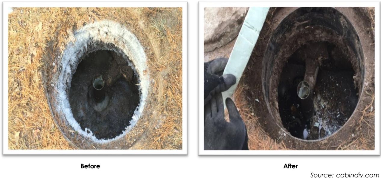
Fig. 4.5: Electric Heating Coil to control frozen condition
