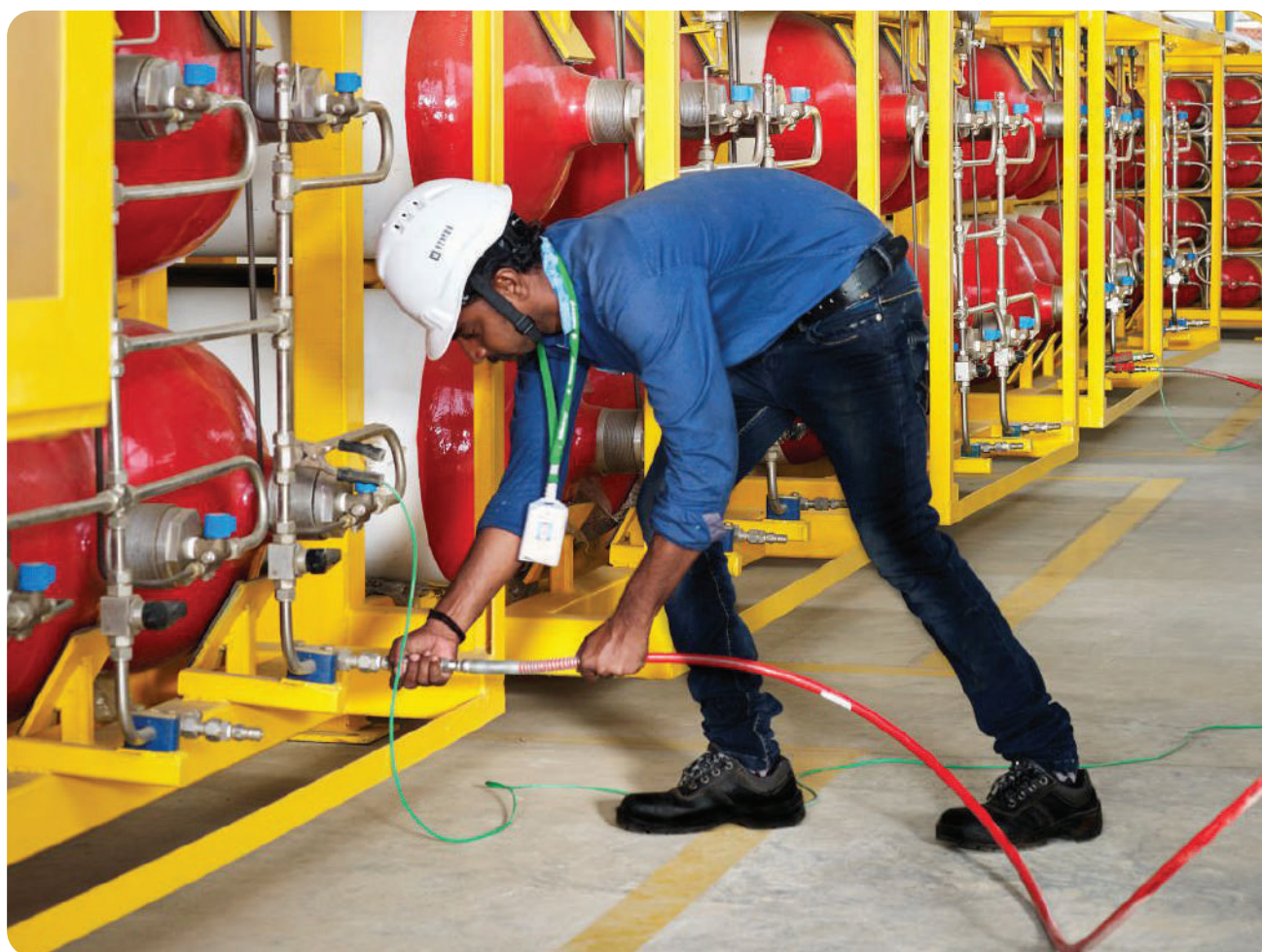
Picture-CBG Cascade at Pune CBG plant
