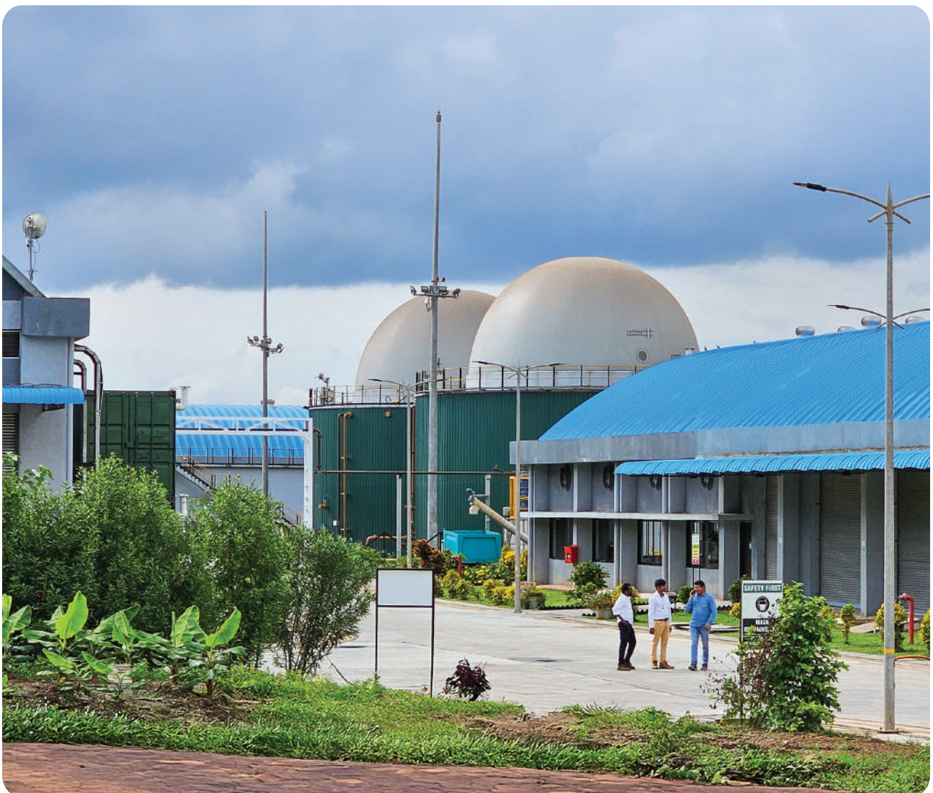
Picture –Biogas Plant, Goa, India
