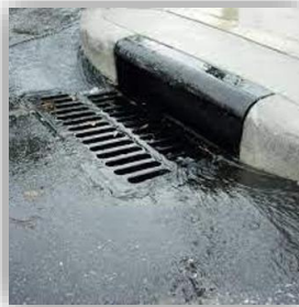
Storm Water Drains
