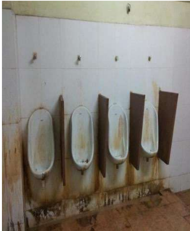
Urinal not clean
