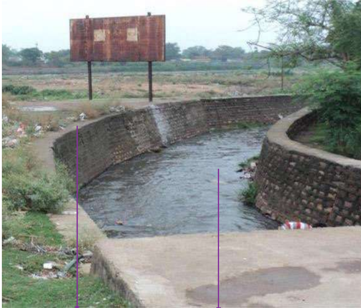
Boundary wall Nallah Without Solid Waste Floating
