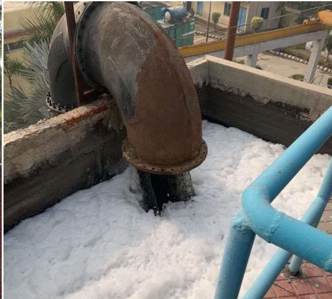
Photograph of inlet sewage
