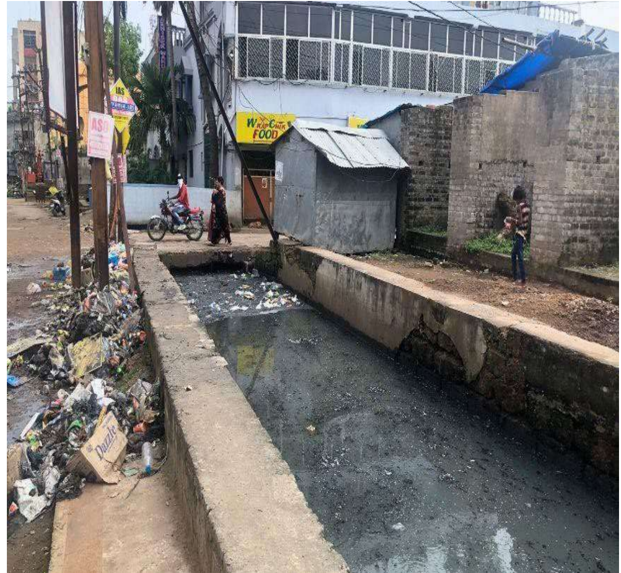
Photograph of SWD with visible/floating solids
