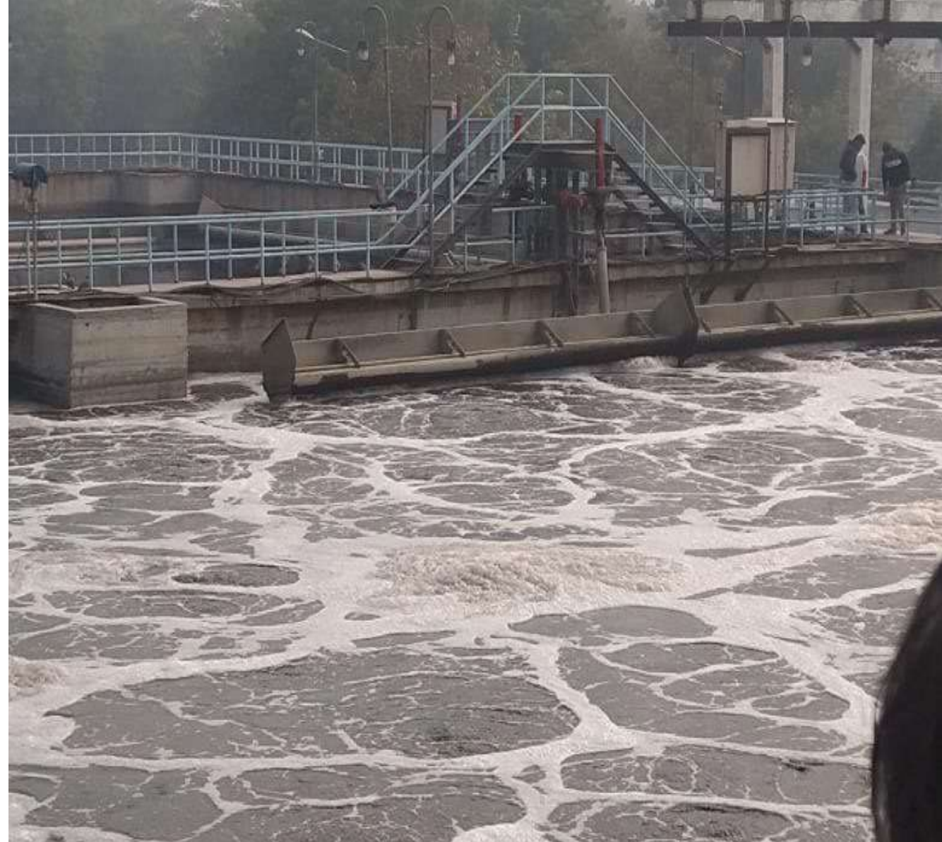
Photograph of STP plant
