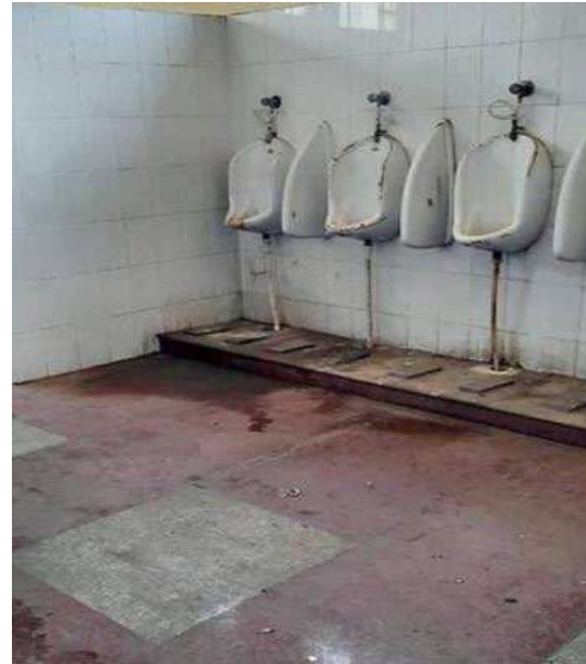
Toilet floor is not clean
